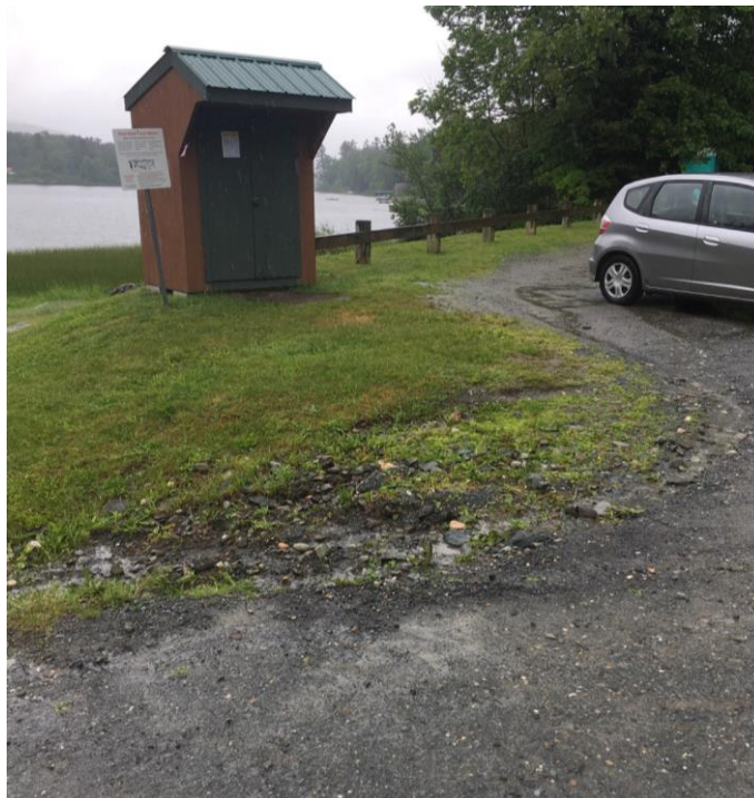
Figure 7: Erosion at the VT Fish and Wildlife Boat access observed during a storm event in June 2019. The concept design for this area (SW-4) describes a BMP that would treat this runoff.
